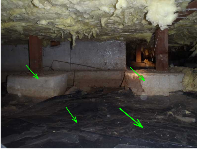
all of crawl is noted with vapor barrier and posts are raised and dry...and solid on piers....
