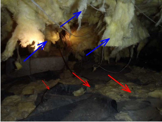
here is past evidence of insulation pulled down by critter infestation...and is also on vapor barrier...remove..
