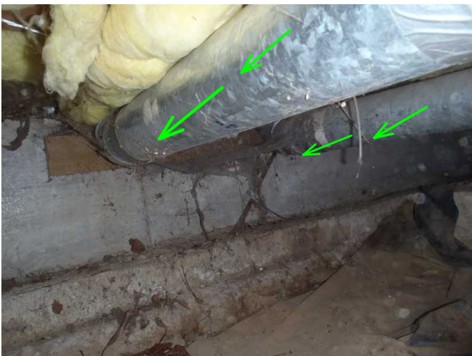
here is back area of home where dryer vents exit and are noted solid and no lint or leaks noted...
