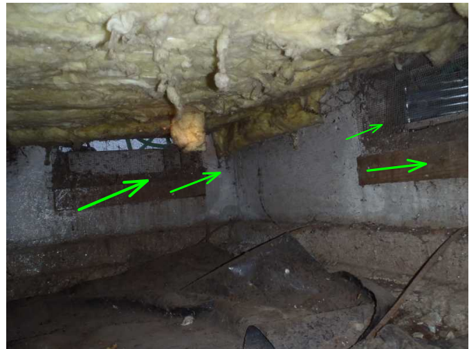
most all the vents are noted screened....monitor all vents to be sure screens are in tact to not allow in critters...
