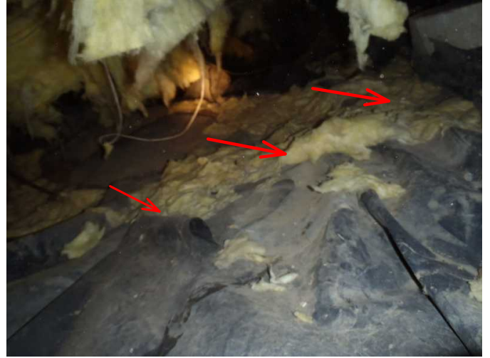
many small areas under structure noted with insulation down on vapor barrier and old critter nesting noted..remove...
