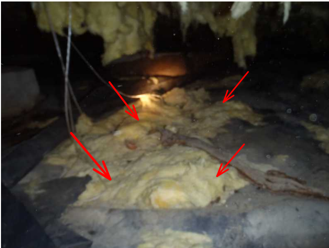
critter nesting is also area where fecal matter and urine is in the insulation..contaminated...remove...
