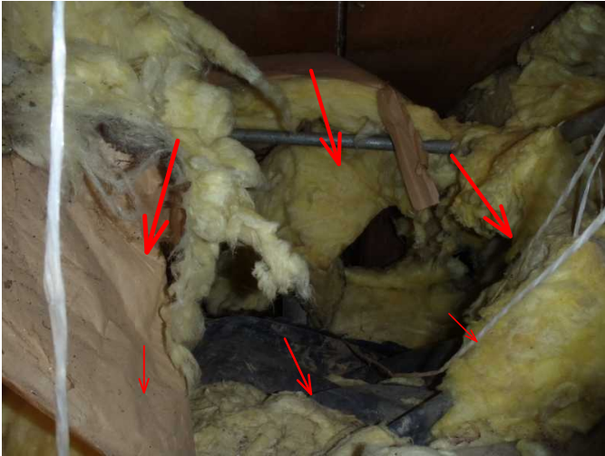
here is area between baths of both units and noted insulation is down and nesting has occurred...remove all contaminated
