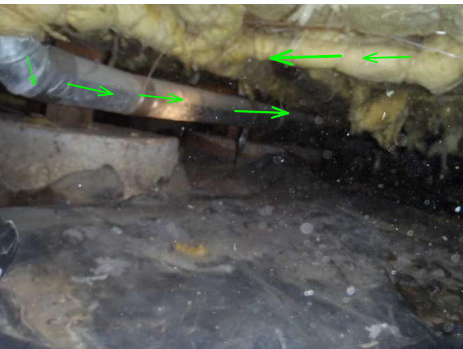
most all water pipes are noted here insulated...and 11900 dryer vent duct is noted solid to exit as well..
