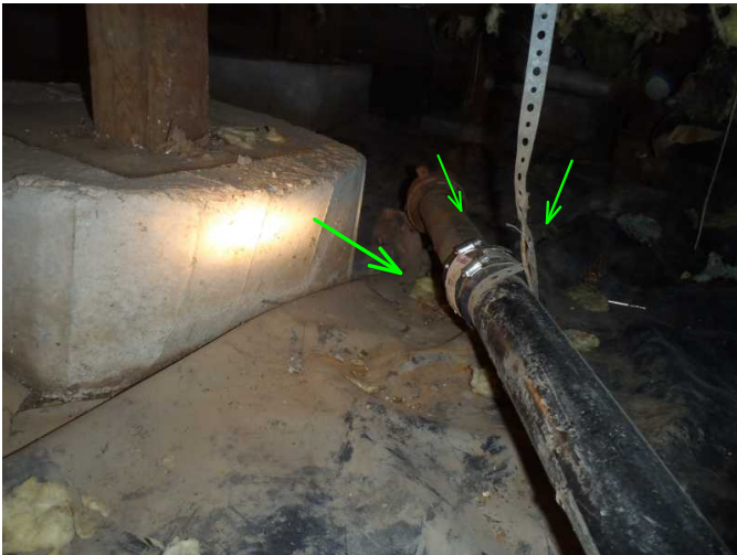
ABS meets original sewer exit drain and is noted clamped as needed...good...no drips or leaks...
