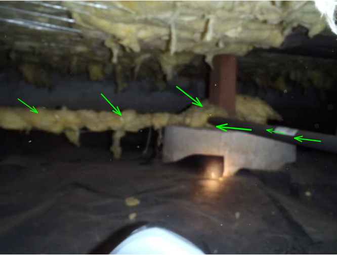
main copper water entry line is noted here and is insulated...good...ABS sewer exit is noted at right center...
