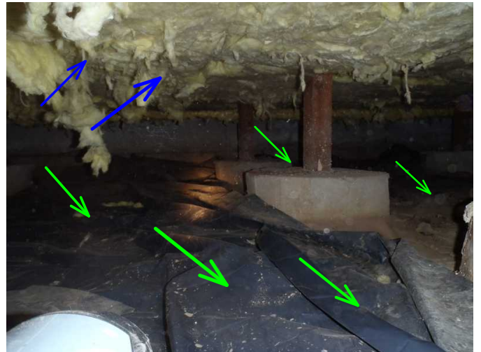
most crawl is noted in very clean and dry condition...posts are raised and vapor barrier in place...insulation shredded
