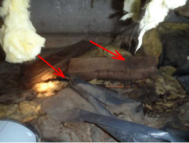
some areas over vapor barrier have wood debris and needs removal...
