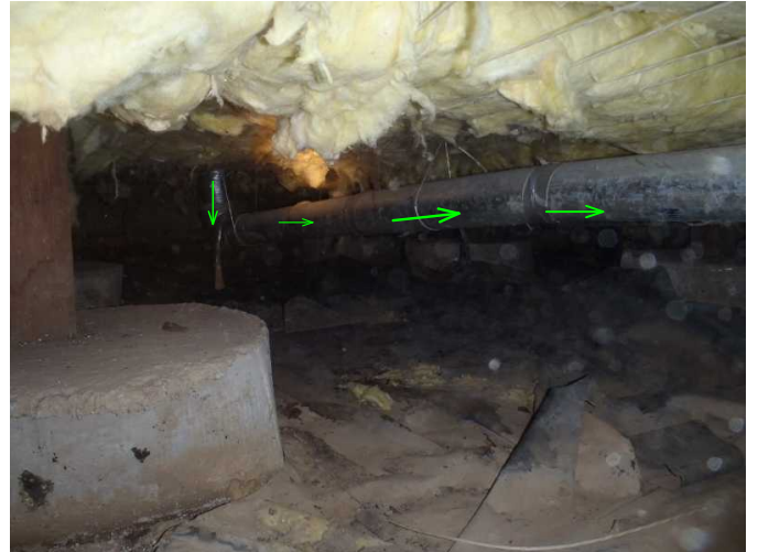
dryer vent is noted with no lint leaks and solid from laundry to exiting area at back of home...
