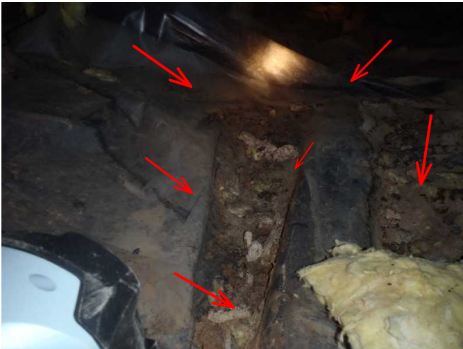
there is also an area where appears is critter toilet area...fecal matter and urine are noted on vapor barrier...remove
