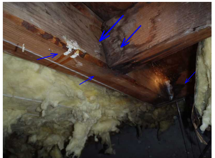
some beams are noted with staining and are noted solid...repairs were performed...
