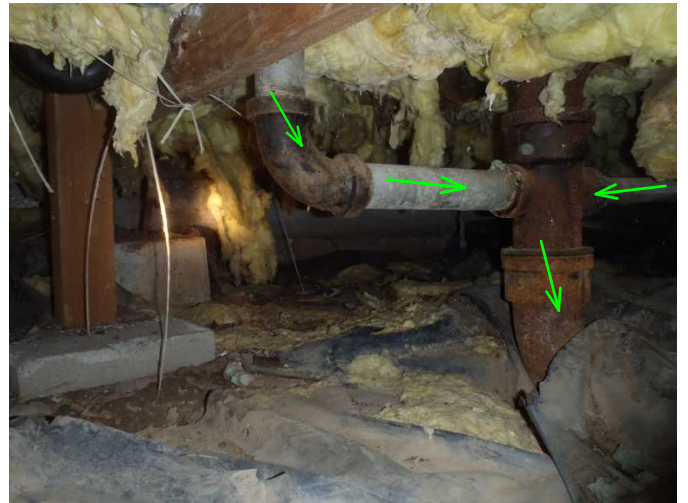
11920 bath exit drains are original and noted no drips or leaks below as well as in area...
