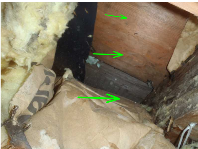
some areas are noted with flooring replaced with plywood under bath areas in 11920 sub floor area where insulation down...
