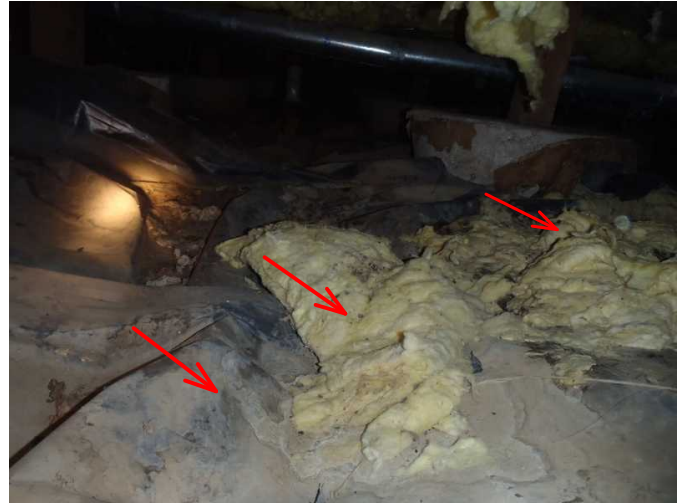
the vapor barrier is noted here with contaminated insulation with critter fecal and urine matter and needs removal..
