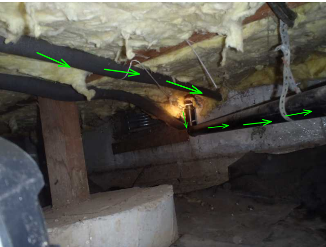
most water lines are noted insulated with insulation or foam...ABS sewer exit lines are noted from both kitchens..newer
