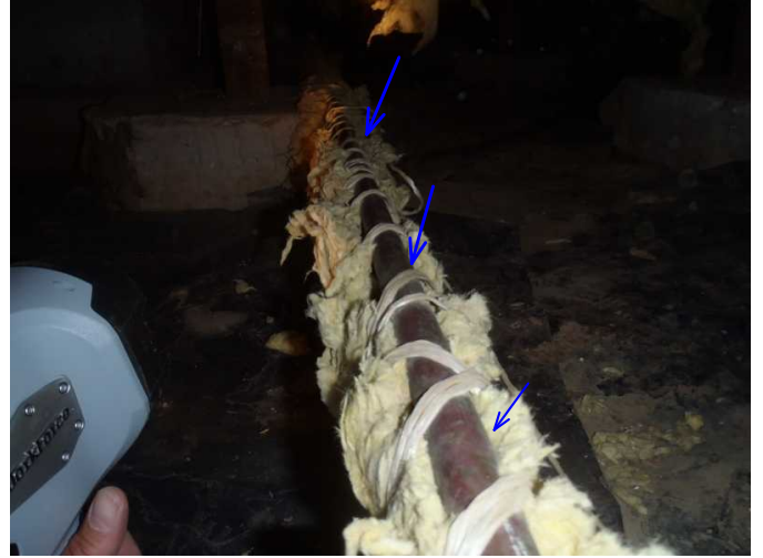
more areas noted that need insulation...main copper water feed lines...
