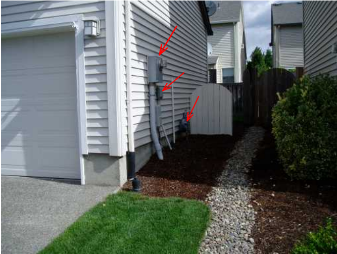
electrical/gas and phone entry at side of garage..all good...
