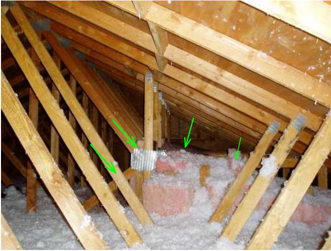
vaulted ceiling above master bedroom has batt insulation...rest of attic is blown..very good job...
