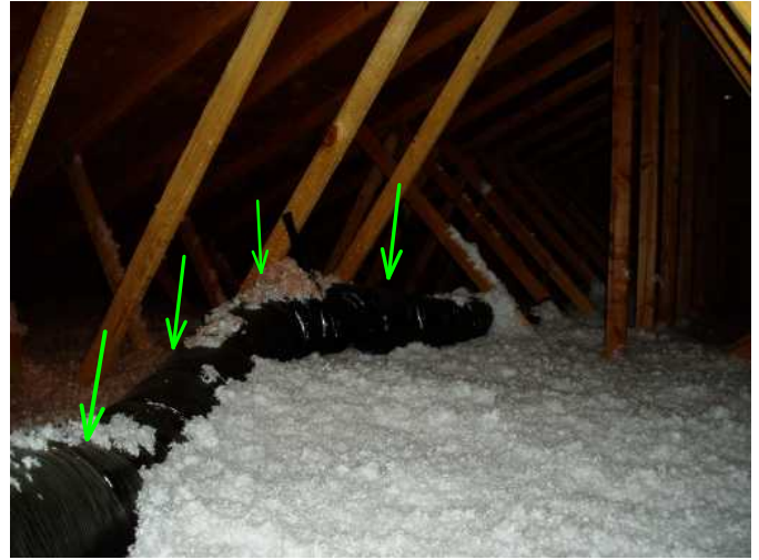
one of several insulducts to various rooms on second floor..good...
