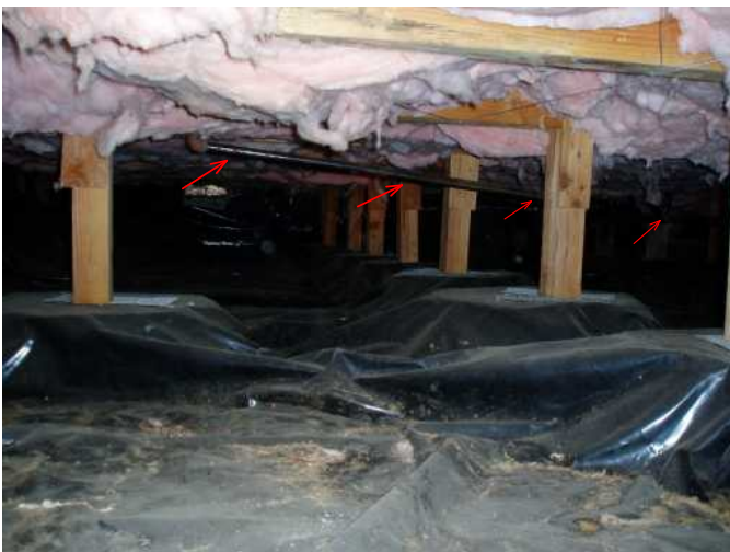
gas service to fireplace is hard piped...
