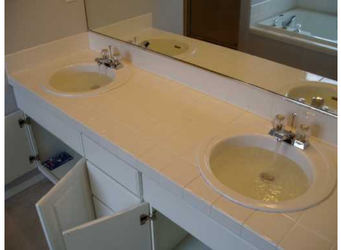
did overflow test on both sinks..did fine...
