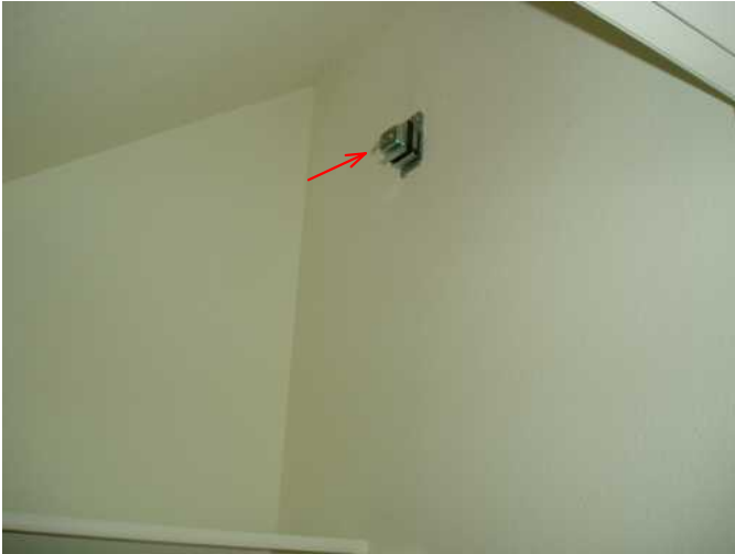
low voltage coverter to operate door bell button in front of home..without shock issues...
