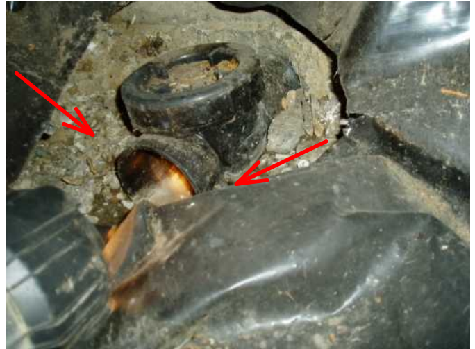
this is exit gate at low corner of crawl floor to let out any water that may enter crawl space..very good...
