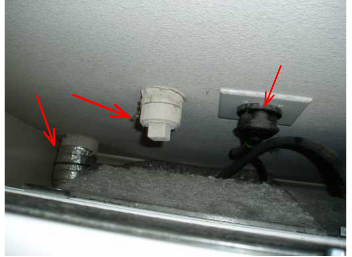
cleanout for drain...dryer hook up and exit duct for outdoors..good...
