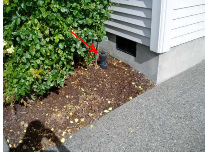
main sewer cleanout..good..
