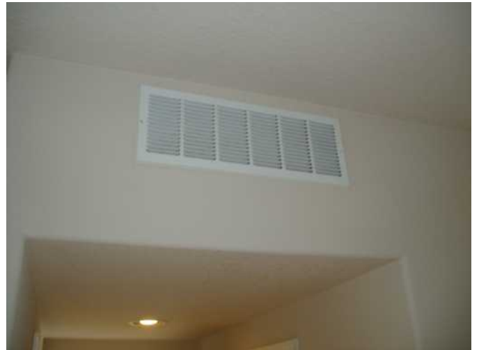
second return air for furnace system in kitchen area..lower level...good...
