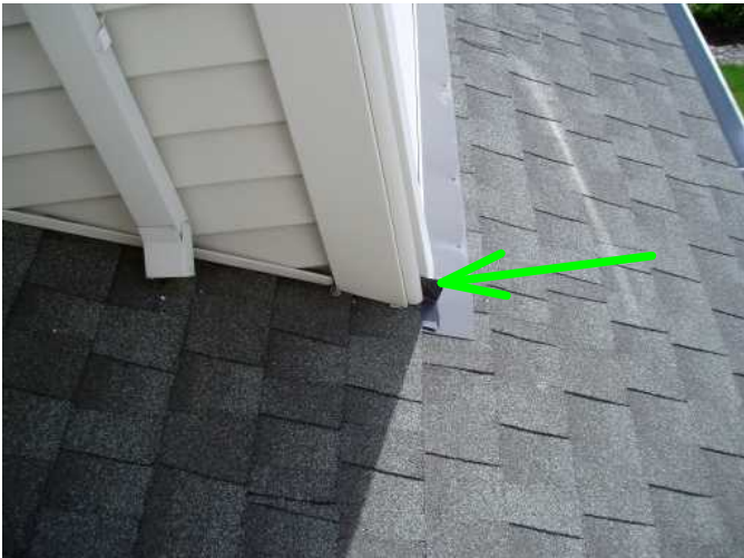
good kickout to keep water from entering under shingles in this area....
