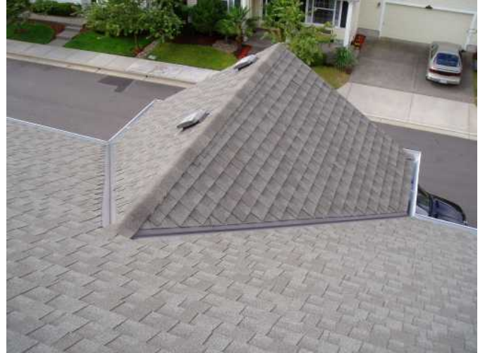
front of roof is vented well ...valley are good...gutters are clean...monitor season to season...
