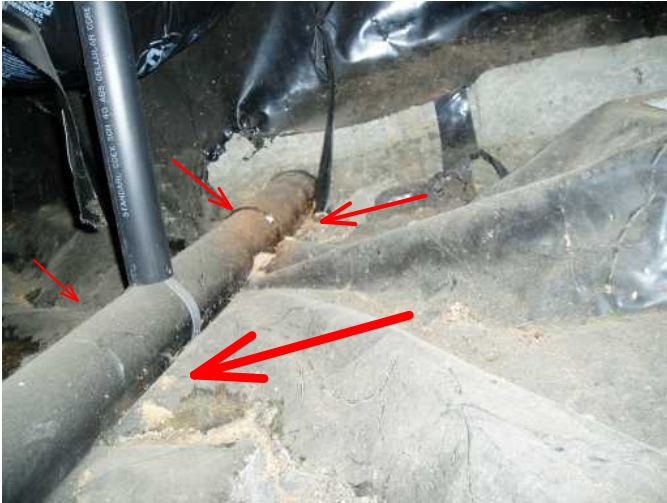
main sewer exit pipe goes out the front of home under dining room...
