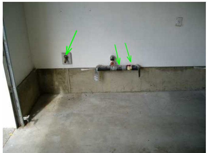
main water entry and shutoff and hose bib with backflow protection..very good....garage...
