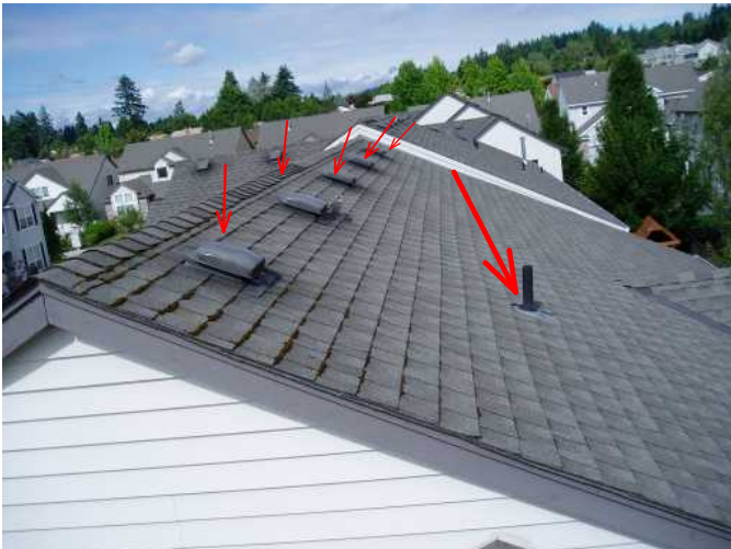
peak of main roof is well ventilated...one of three sewer exit vents to keep sewer pipes flowing...good...
