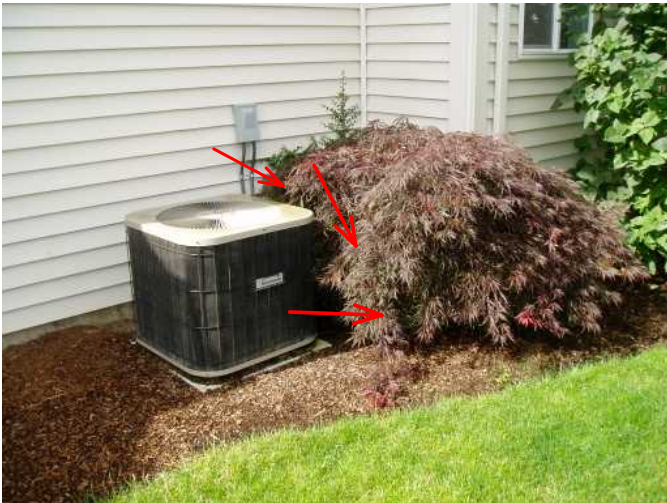
a/c unit was installed after home was built..runs fine..trim back shrub here is to close to unit to make it work harder.
