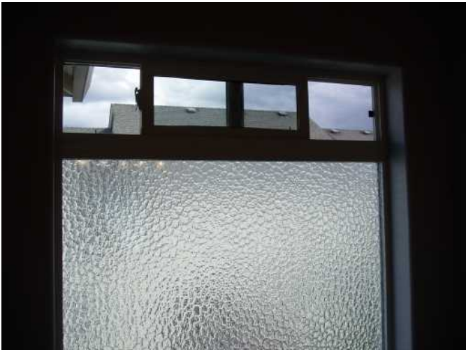
upper window worked fine above tub..master...
