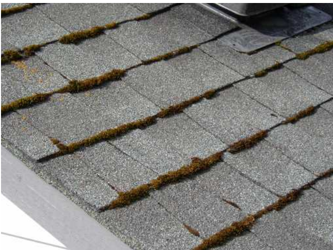
this is moss on upper rear side of roof..appears to be treated..will need treatment every year..is normal...just monitor
