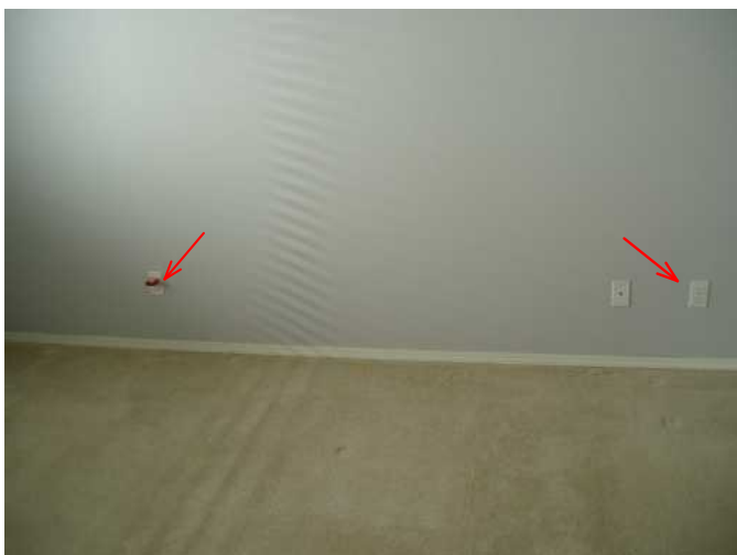
master wall outlets are switched for lamps..good...
