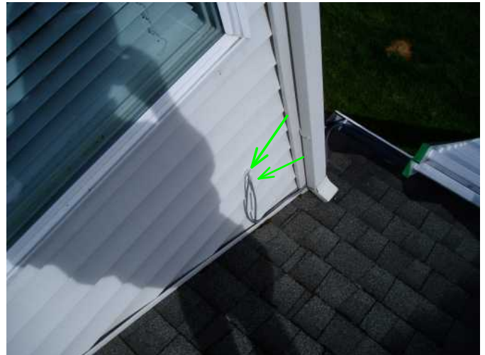
dish type television cables are installed well with grommets to keep out water....
