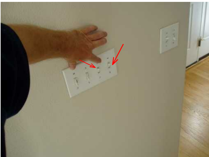
could not determine what the two right light switches in dining room operate...please have seller disclose...
