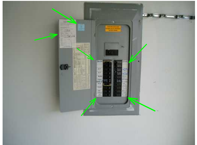
electric panel open showing well marked for zones and has permit sign off and blue tag for a/c installed later....good
