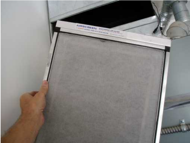
furnace filter is electronic and is replaceable insul fiber ..see directions on side of furnace....
