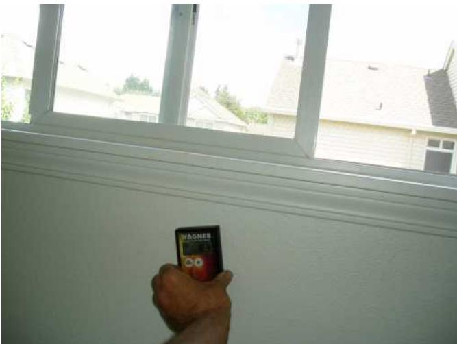
master closet window worked fine...did moisture check of walls around windows and at random, 5.5% - 7.7% good...
