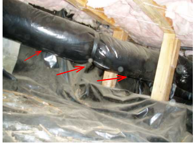
all insulated duct work is in tact and connected and performing well....
