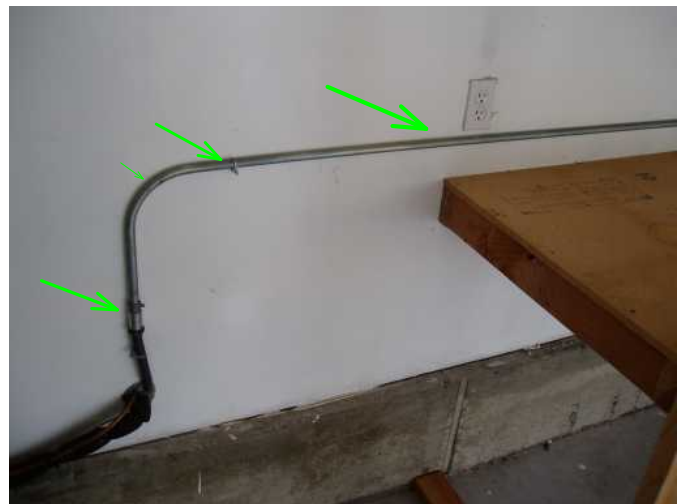
newer a/c electrical service is in conduit ..very good...
