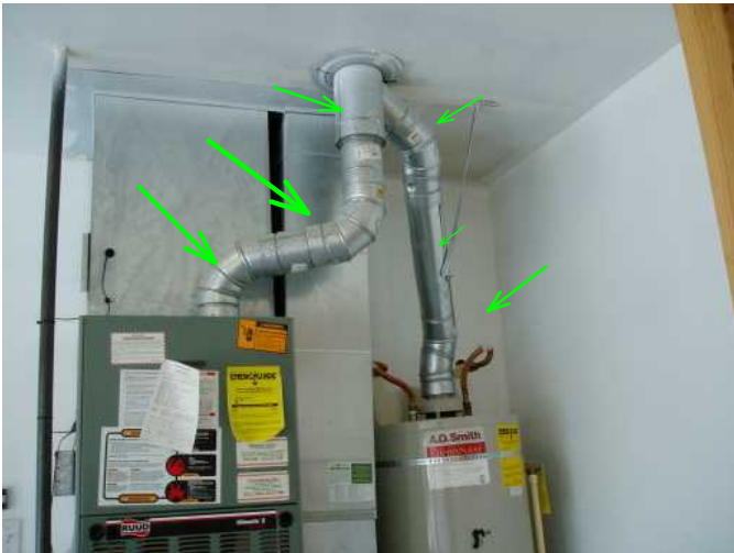
exit flus are installed well and solid....
