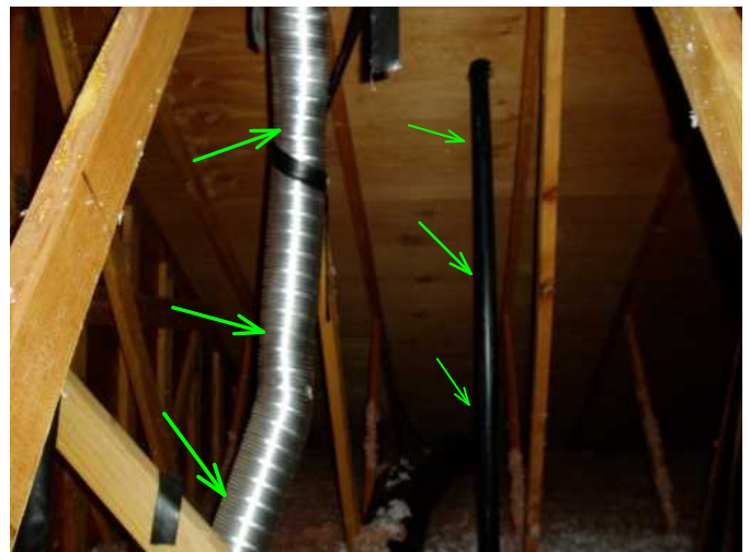
attic is plywood sheathing and 2x4 truss system...bath venting is good from both baths...one sewer vent pipe noted here.
