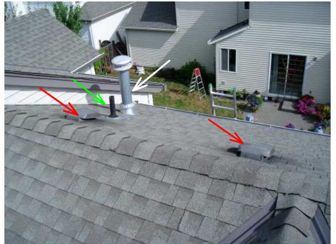
red more roof vents ...good...white ...exit flu for furnace/water heater...good...green..sewer vent pipe in action..good
