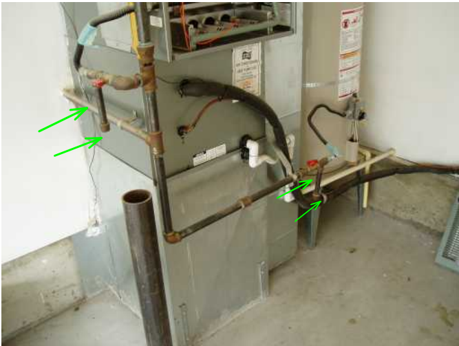
gas service to furnace and water heater are installed well and solid..have two drip legs to catch impurities in the line
