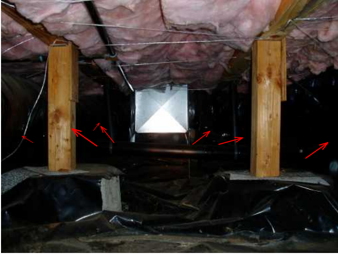
main distribution of furnace/a.c system at garage side with insulated duct running throughout crawl space....good...
