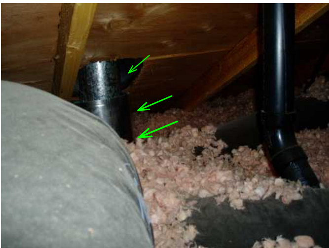
this is furnace and water heater exit flu with attic shield to protect pipe from insulation..by the book...good...
