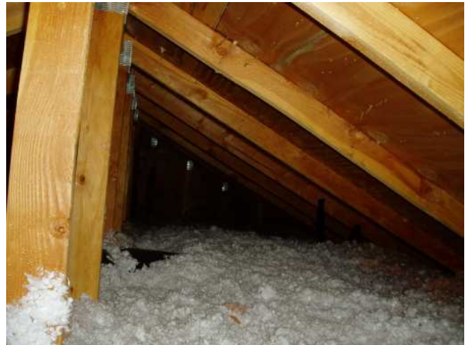
lower attic area above great room on right side of home..lower attic area...good insulation here too...
