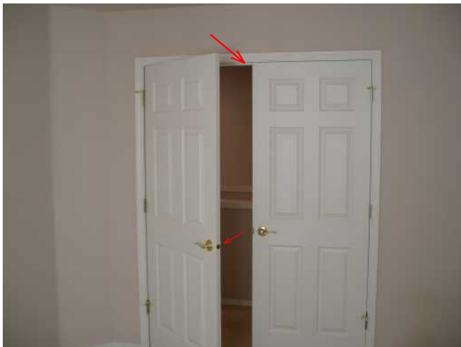
exit doors to hallway are operable and attach to frame fine...latch properly...
