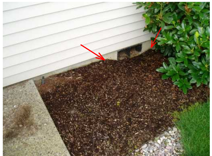
this is vent with too much barkdust and will allow rain water entry to crawl space...keep even or below vent opening
