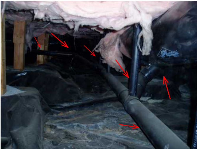
main sewer exit pipe is solid and sound with no leaks noted....
